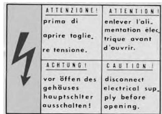
Electrical warning Adjacent to the master switch
